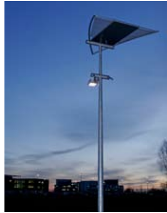
Solar powered lighting on Moston Vale
